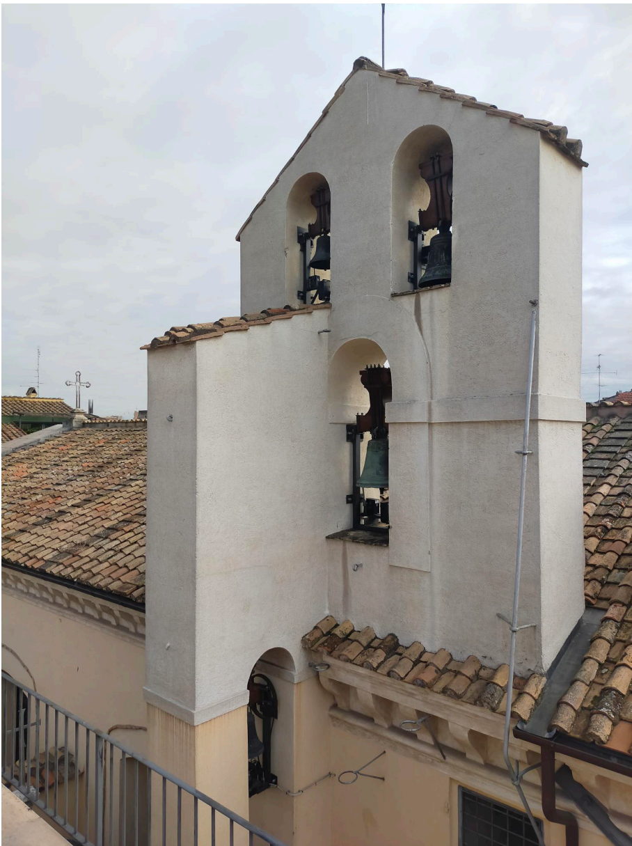
Fig. 3. Bell gable of Santa Maria in Monserrato degli Spagnoli, with four openings for bells. The author
